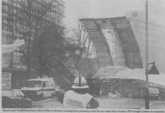
Ripped apart: Scaffolding from a block of flats in Belston crumpled down yesterday as the fiercest winds since October 1987 brought London to a standstill.
